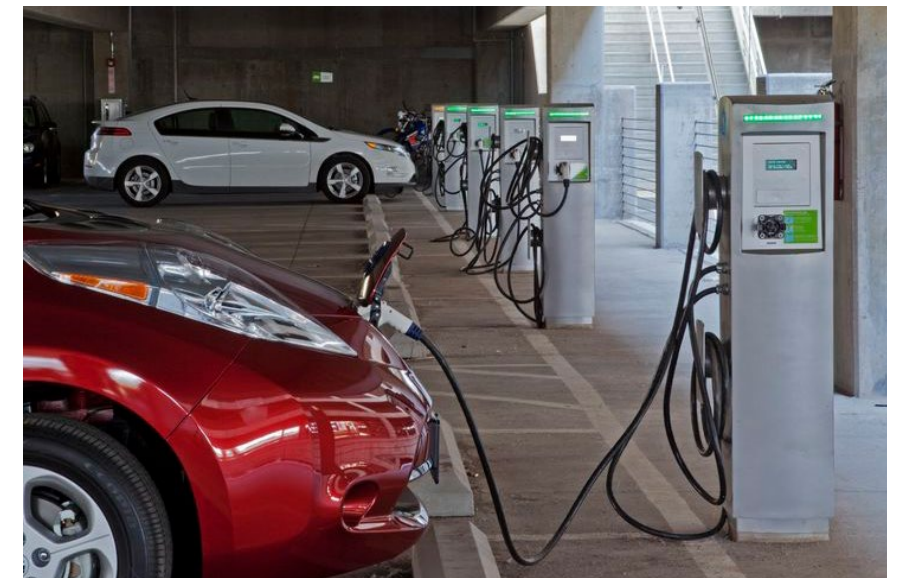
I3(b) Electric Car Recharge Facility
